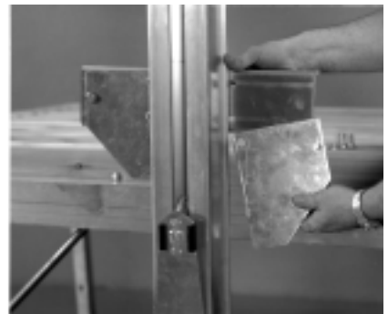
18. Mount one (1) hoist attach plate to the winch post mounting channel using three (3) 3/8" X 1" carriage bolts. Secure with 3/8" flange lock nuts. NOTE: The hoist attach plate must be hooked over the lip on the winch post extrusion. Place the other hoist attach plate onto the opposite side of the winch post extrusion - be sure this plate extends over the lip of the winch post extrusion before tightening.
